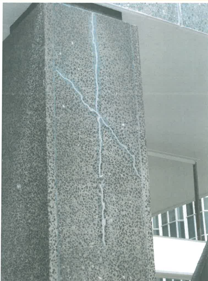
Fig.4 - Angular cracking alignment.
